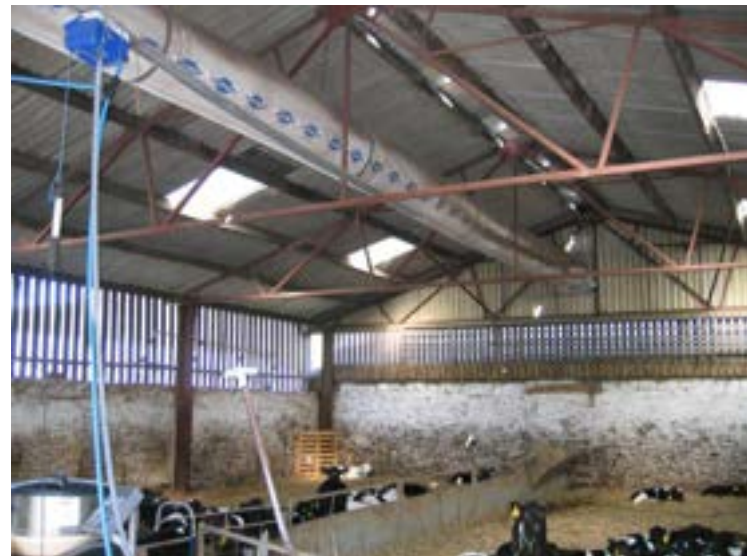
'Positive pressure tube ventilation'
