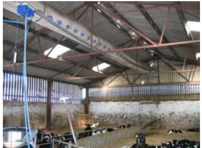
Positive pressure tube ventilation
